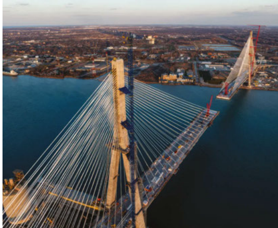
PHOTO CREDIT: PATCH, BRIDGES & TUNNELS
